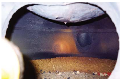
The result of oil contamination in an oil-fired boiler.
