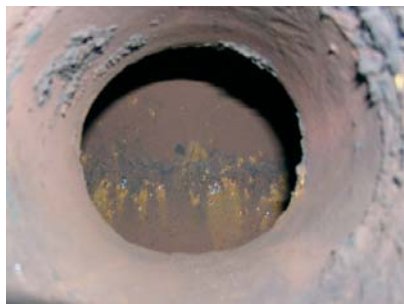
Severe pitting and scaling in downcomer tube
