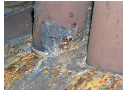
Corroded boiler furnace dome and convection tubes
