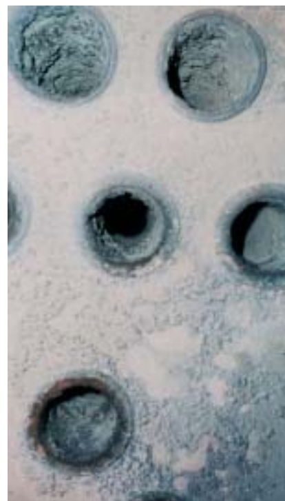
Boiler scaling of tube plate and tubes
