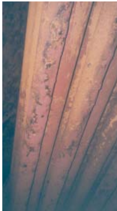
Boiler scaling on boiler tubes in composite boiler
