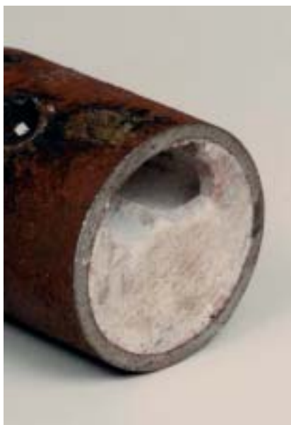
Boiler scale on water side
