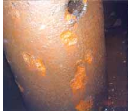
SUNROD™ pin tube damaged by oxygen corrosion (pittings).
