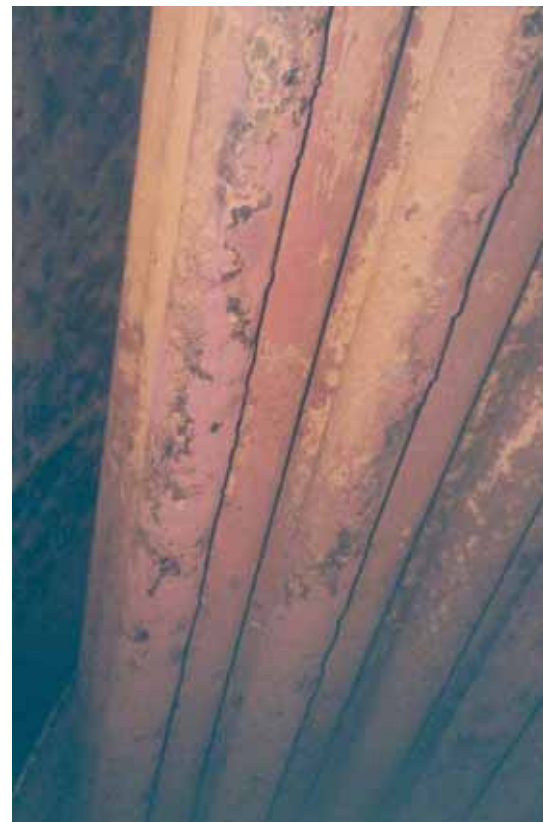
Boilers scaling on boiler tubes in composite boiler
